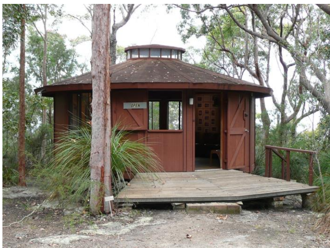
The Katandra yurt and the veranda platform that has been in need of repair. The tree to the left of the platform is an Angophora costata .
